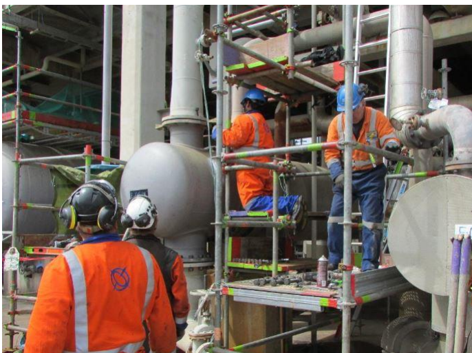
Distillation Plant – Heat Exchanger Assembly
